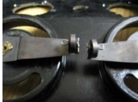
Photo #12 Roller arm clearance.
