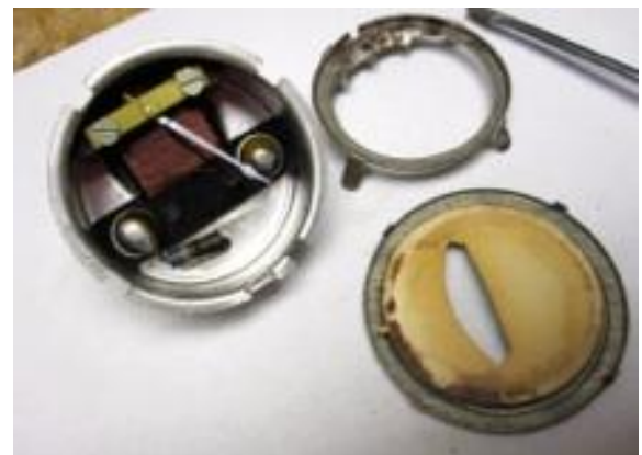
Photo #15 Disassembled meter
